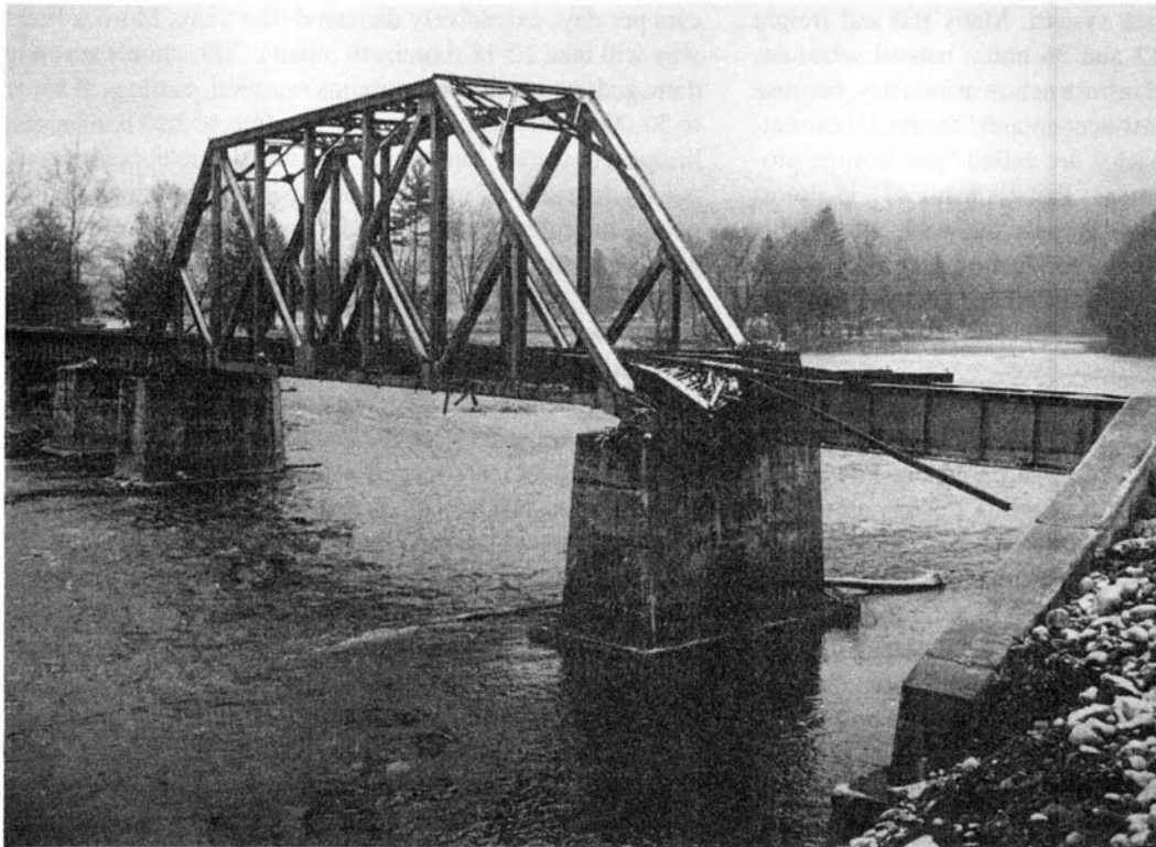
A bridge in West Virginia. The collapse of U.S. infrastructure of all types, as a result of the insane policies of free-market economics, has created catastrophes just waiting to happen.
