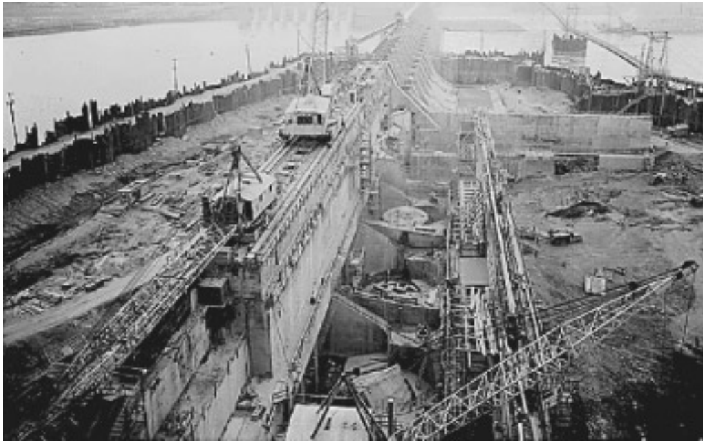
Construction of a dam and power plant by Roosevelt's Tennessee Valley Authority in 1942. Such state-organized public works can supply an effective degree of relative (Riemannian) physical-space-time curvature to the domain within which the relevant private enterprises are situated.
