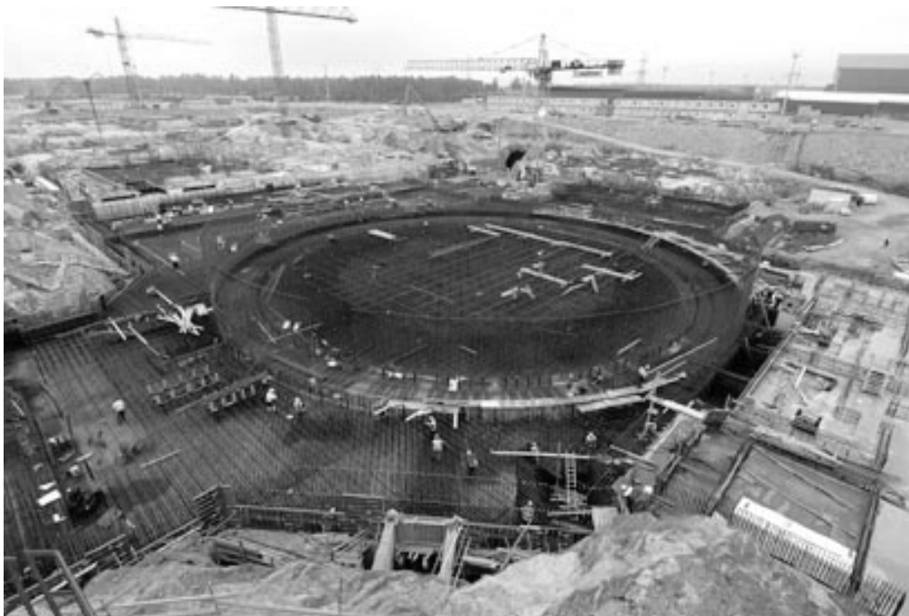
The U.S. nuclear manufacturing capability has declined greatly over the last 30 years, but the super-sized 1,650-megawatt-electric generator for the Evolutionary Pressurized Reactor nuclear plant that Areva is building in Finland (shown here), is being made in the Siemens facility in Charlotte, N. C.
