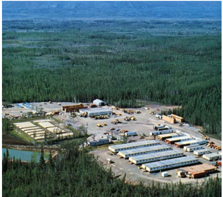
The base camp for an oil pipeline construction project across the Yukon River, at Five Mile, Alaska. For NAWAPA, the headquarters would be something like Mission Control for the NASA missions.
