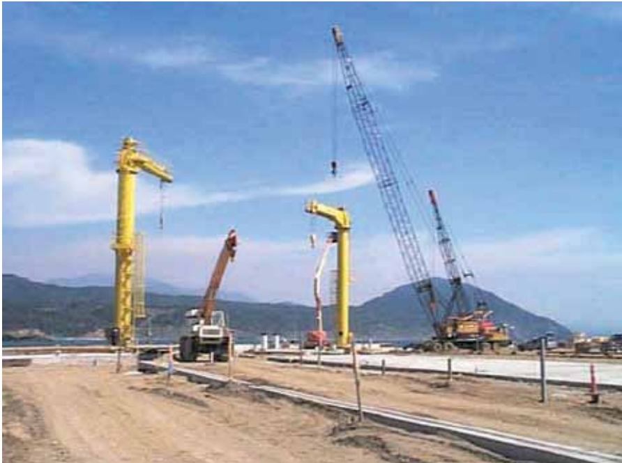
Among the African projects which China is involved in, is the Lamu Port and South Sudan Ethiopia Transport (LAPSSSET) Corridor, shown here under construction. The huge project involves building a modern port at Lamu on the Kenyan coast, not far from Somalia, along with an oil refinery.
