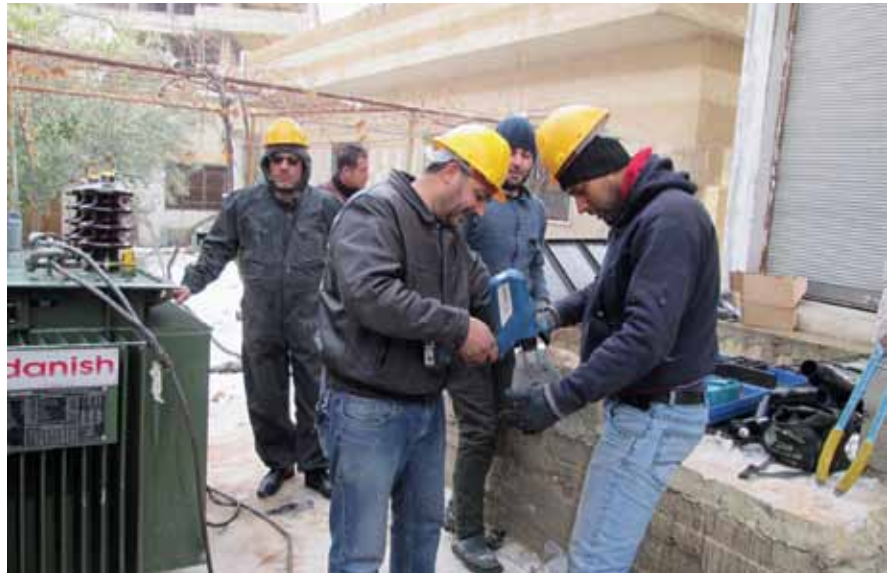
Electrical workers at work in the suburbs of Damascus. Repairing the electricity grid will be a major task of reconstruction.
