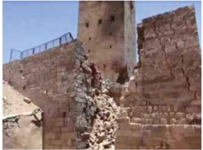
Fig. 16 Detail of a floodgate of the dam, damaged by air raids.
