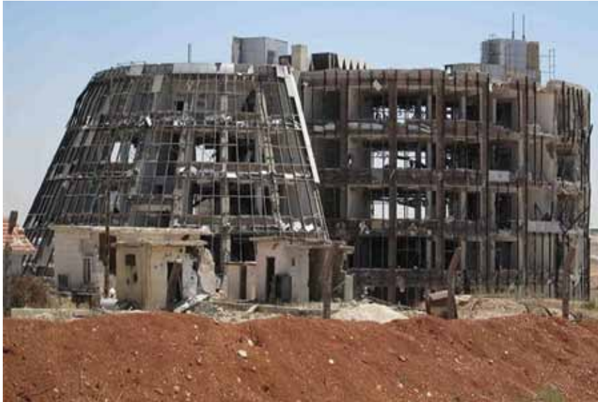
Damaged building in Sheikh Najjar Industrial City, near Aleppo, Syria.
