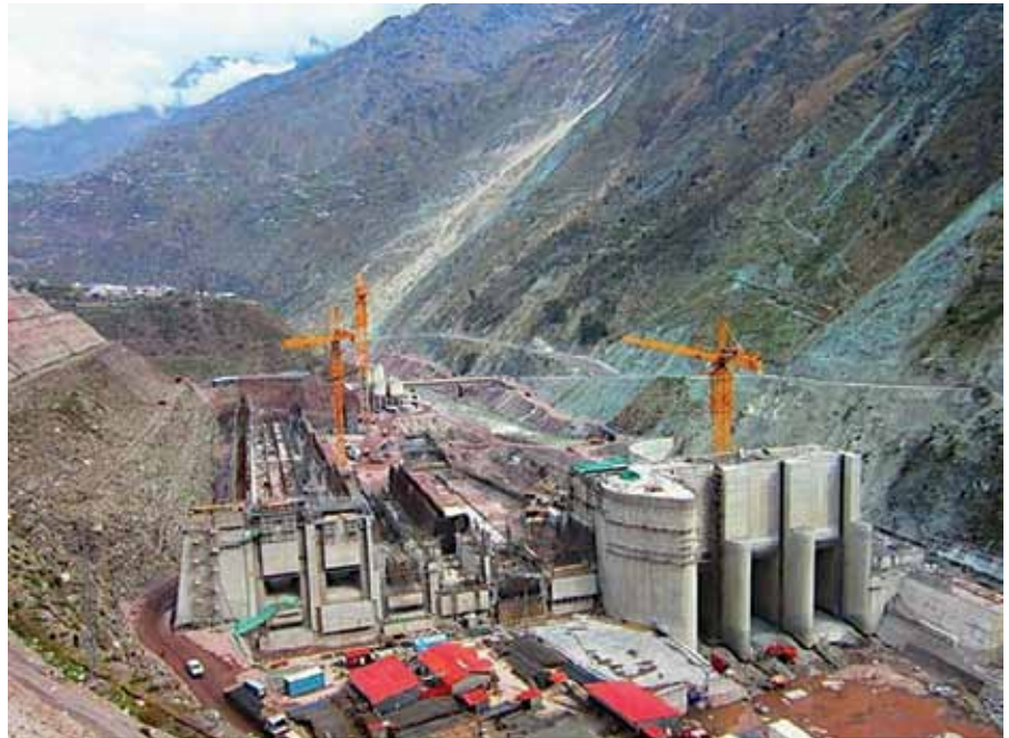
Neelum Jhelum hydro power project while under construction in Neelum Valley, Azad Kashmir.
