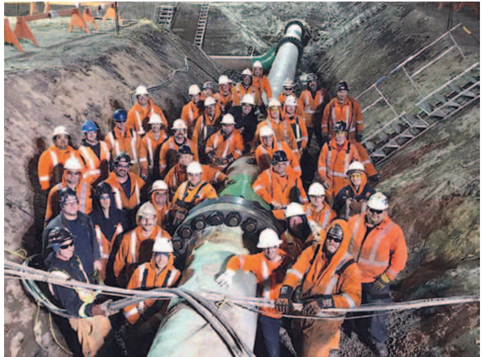
Enbridge crew at the Gretna, Manitoba Terminal stands by the southern end of the Canada Line 3 Replacement pipeline.
