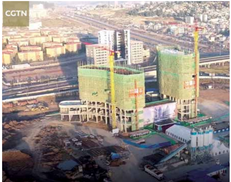
The future headquarters of the Africa Centers for Disease Control and Prevention (Africa CDC), in Addis Ababa, Ethiopia, under construction by the China Civil Engineering Construction Corporation, Nov. 29, 2021.
